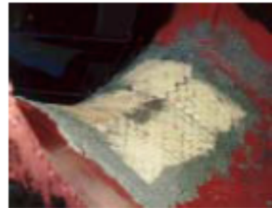
'DILLO HYDE™ used to repair contoured discharge area of exhaust fan housing.
